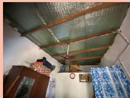
Heat-reflective foil installed under the ceiling is a more costly yet effective solution seen in Colombo.
